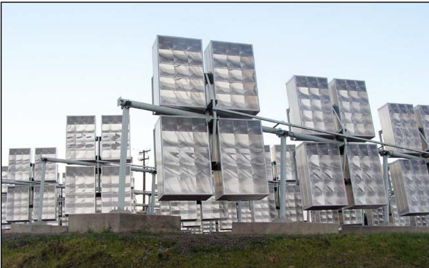
Maui, Hawaii – Gen3 CPV Installation
