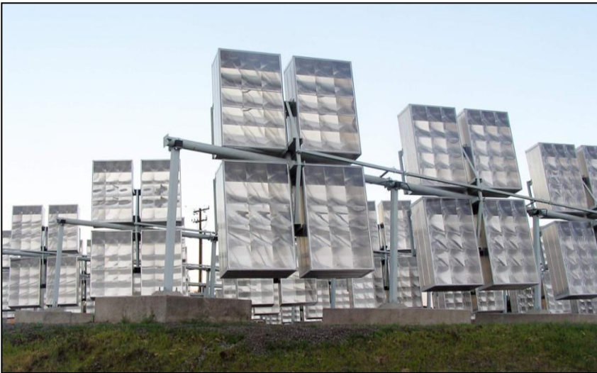
Maui, Hawaii – Gen3 CPV Installation
