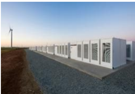
South Australia Energy Storage Project
