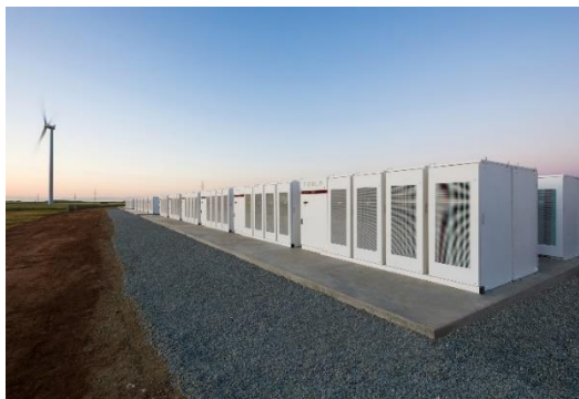
South Australia Energy Storage Project
