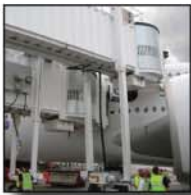
Passenger Boarding Bridges
